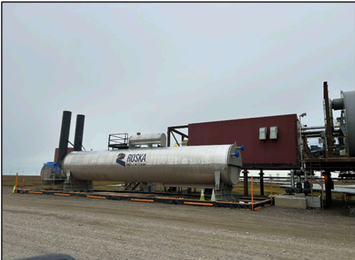
Rental Line Heater LH41 on site in Alaska
